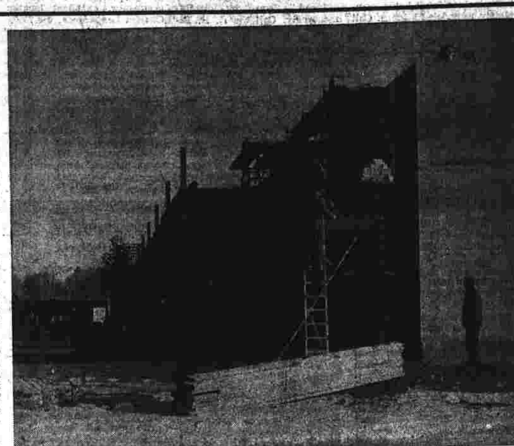
Workmen are shown erecting the steel framing to the front of the new Broad St. Parkade building on the west side of Broad St. The massive building covers an area the size of five football fields. Fifteen to twenty stores will occupy the space and the main tenant will be King's, occupying 70,000 square feet of the building. To the rear of this structure will be built a new theatre which has recently been leased for 20 years to Cinema East Inc. The building pictured is scheduled for completion early this spring. (Herald photo by Pinto.)
